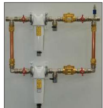
Duplex parallel final filtration
